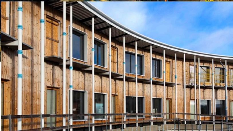
The façades have been installed, and the silver Kalzip roof is taking shape and will be completed in spring 2024.
